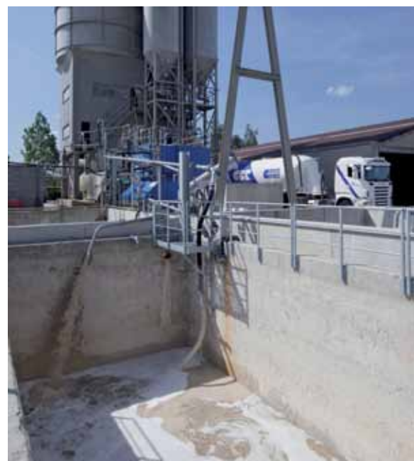
Water Recovery System + bij Inter-Beton in Dendermonde.
